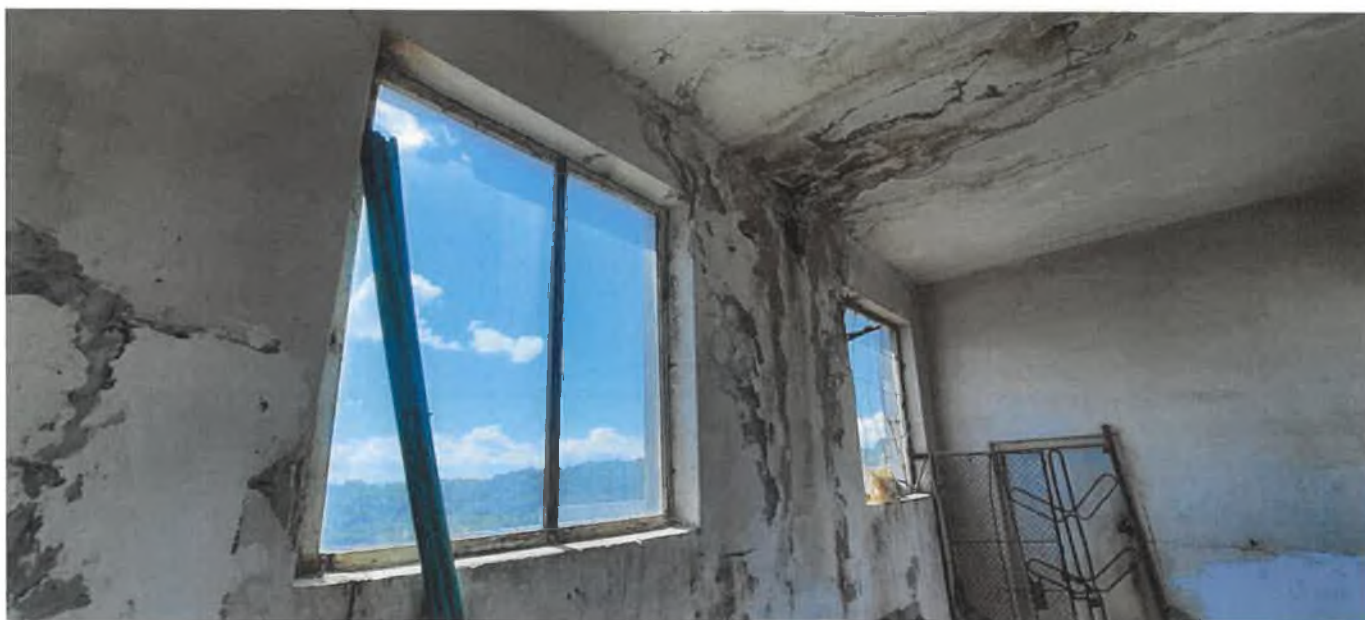
Infiltratii casa lift - terasa
