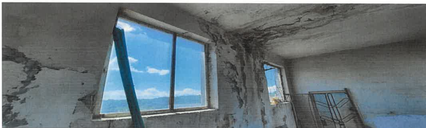
Infiltratii casa lift – acces terasa
