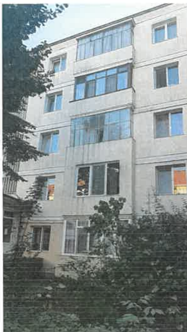
Inchideri balcoane fatada principala neconforme
